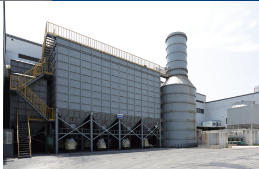
环保设备区 Environmental protection equipment area
